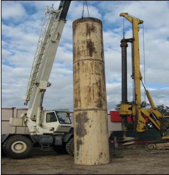
Photograph 1: 30-foot LDA casing with crane for casing the LDA holes from 20 to 28 feet bls.
