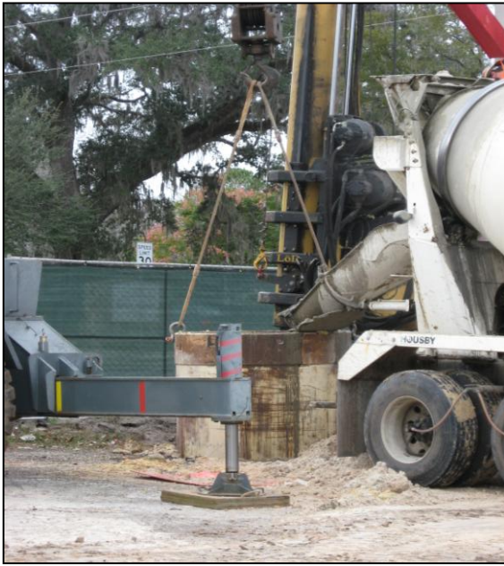
Photograph 5: Fill is added to the boring as the casing is removed to ensure that the formation does not flow into the boring void.
