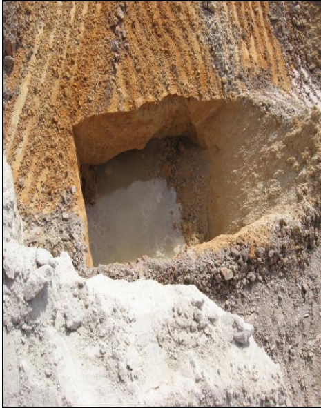
Photograph 1: Test pit to determine static water table (~17 feet bls) for setting dewatering pumps.
