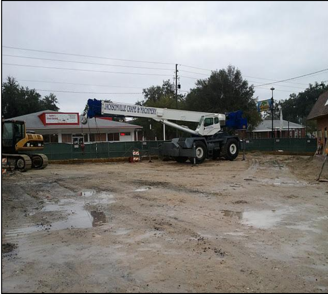
Photograph 1: Heavy rain occurred 1/17/12. No work was conducted other than checking stormwater controls.
